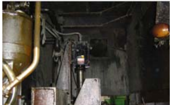
Exit of Cold Rolling Mill
